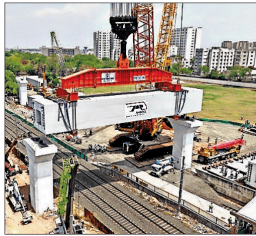
The precast concrete structure measures 34m in length. Five such beams are planned in the vicinity of Maninagar railway station
